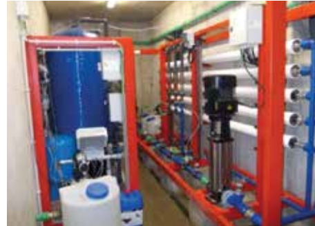
Water treatment system composed of ultra filtration and reverse osmosis system.
