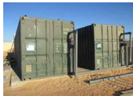
Compact effluent treatment plant.
