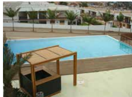
Technical assistance for the maintenance and control of the pool water treatment system.
