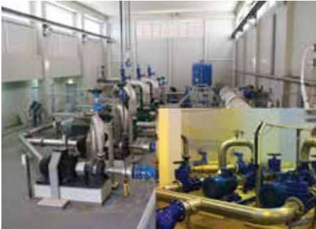
Pumping stations for water supply.
